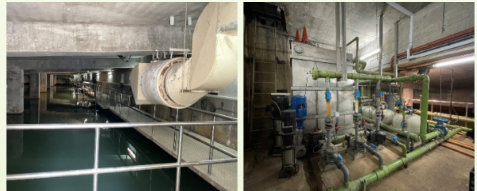
Underground rainwater harvesting system
